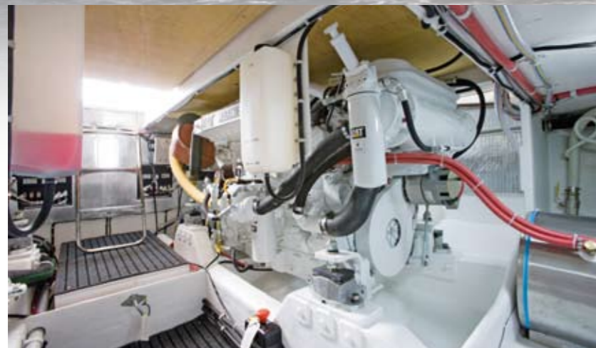
A floorhatch in the saloon leads below to the engine room (left), where there's servicing room all around the two CAT engines. Among the options on the test boat was a neat-fitting washer-dryer (below left).
